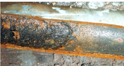
Figure 1. Scale and corrosion as shown above are minimized with regular and accurate measurement and treatment.
